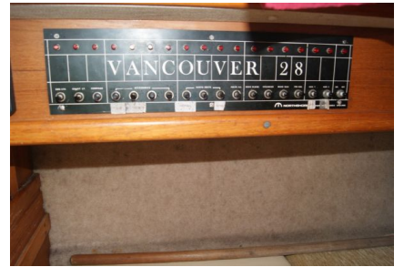
Vancouver 28 - Electric Panel
